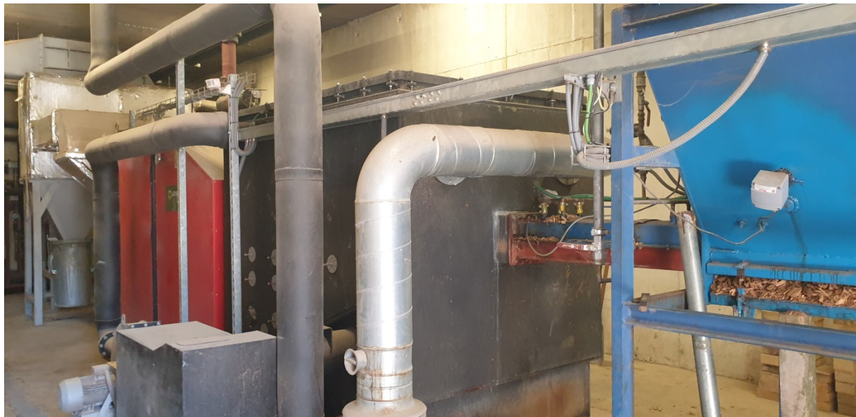
Boiler Room with supplying hopper
